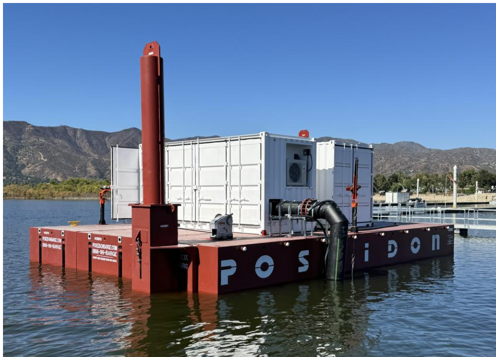
Figure 3: System Installation Picture
