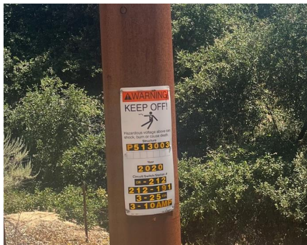
Figure 2-11. Power pole structure P513003
